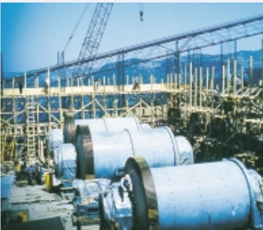
Delivery and installation supervision of 4 copper ore grinding mills, \varnothing 5.3 x 7.8 m.
