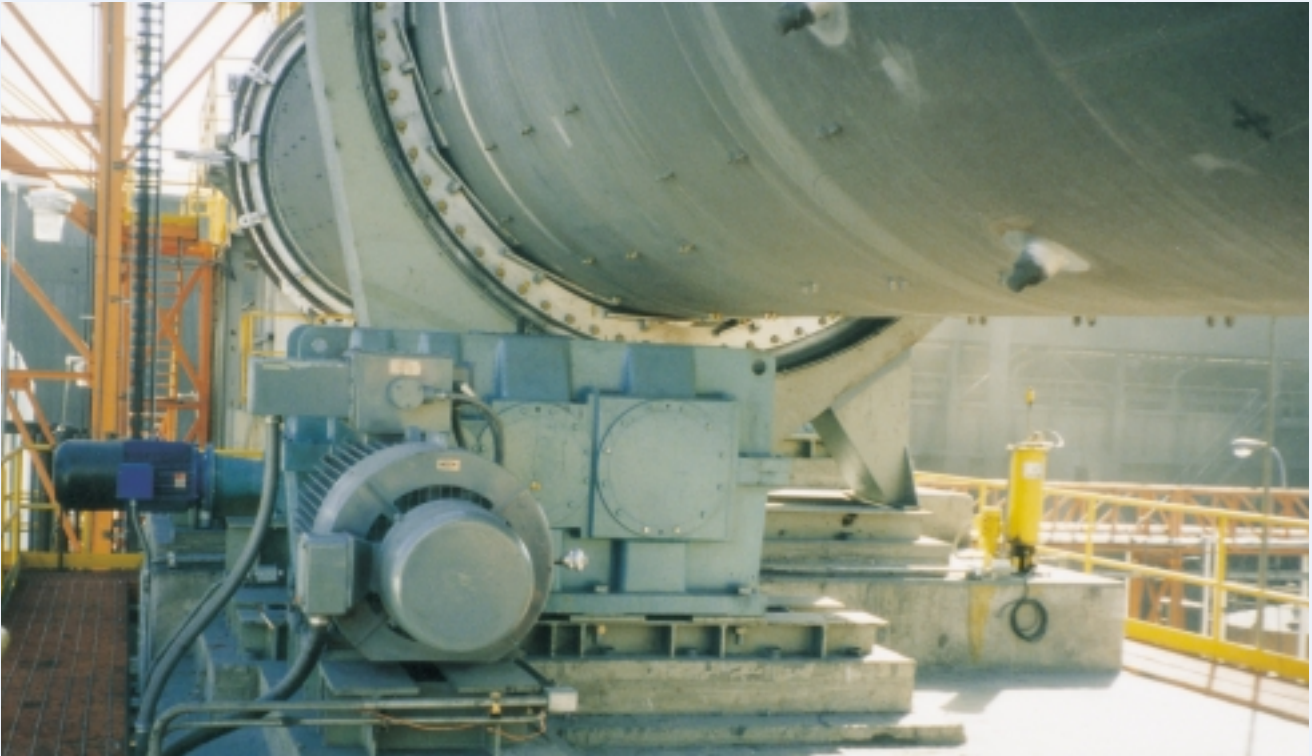
A rotary dryer for copper concentrate driven by Kumera gear LD-4630E with maintenance drive KFA-3140. Drum \varnothing 3.6 x 38 m, capacity 160 tons/hour.
