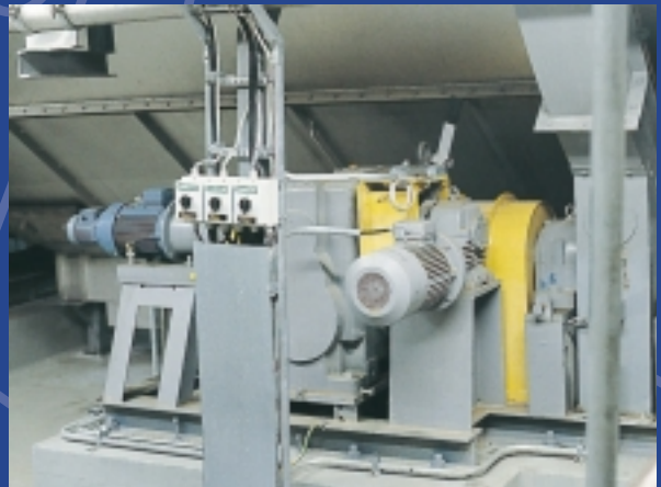
A drive unit for a kiln burning hazardous waste.
