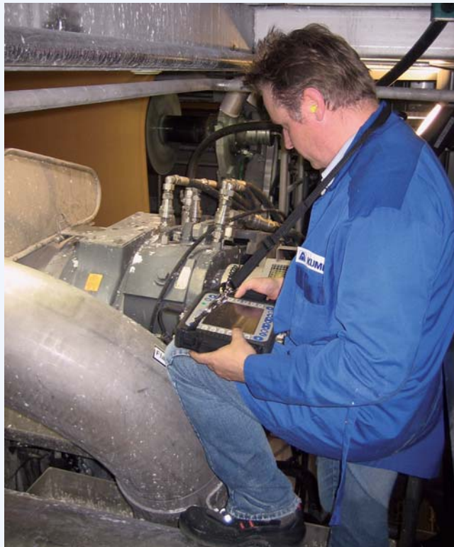
Kumera Drives provided start-up supervision of the integrated roll drives in September 2006. The Project Manager measures vibration with the spectrum analysis device.
